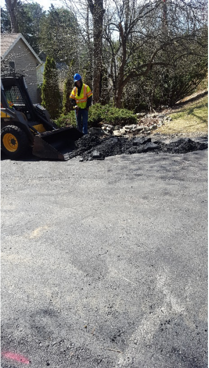
Unsatisfactory curb removal on the south side of the street.
