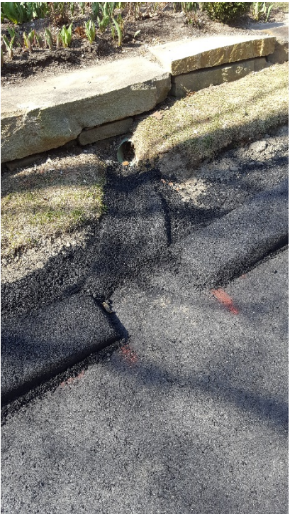
Paved swale to catch roof drain on the south side of the street.
