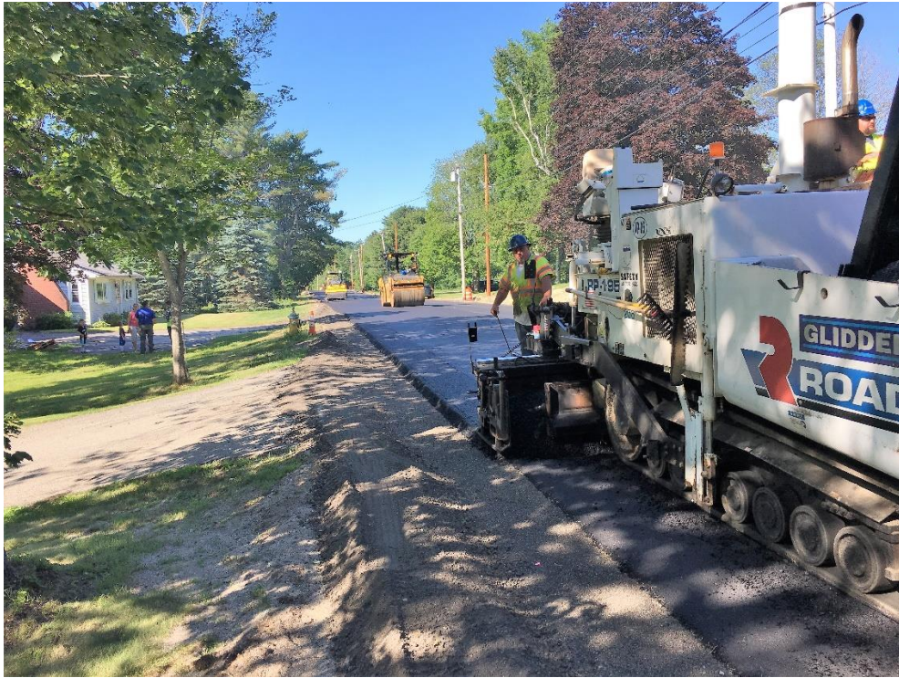
Paving 2 nd layer of base pavement in the northbound lane in northerly directioning.
