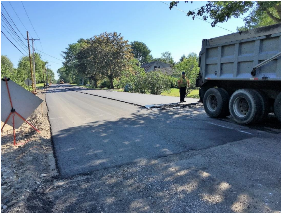
Installing a temporary paved ramp for the northbound lane at STA 62+00 prior to switching over to pave the southbound lane. A similar ramp was installed when the southbound lane was completed.
