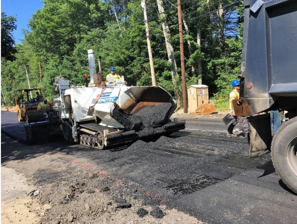
Changing trucks just before paving into the butt joint in the northbound lane at STA 79+00.
