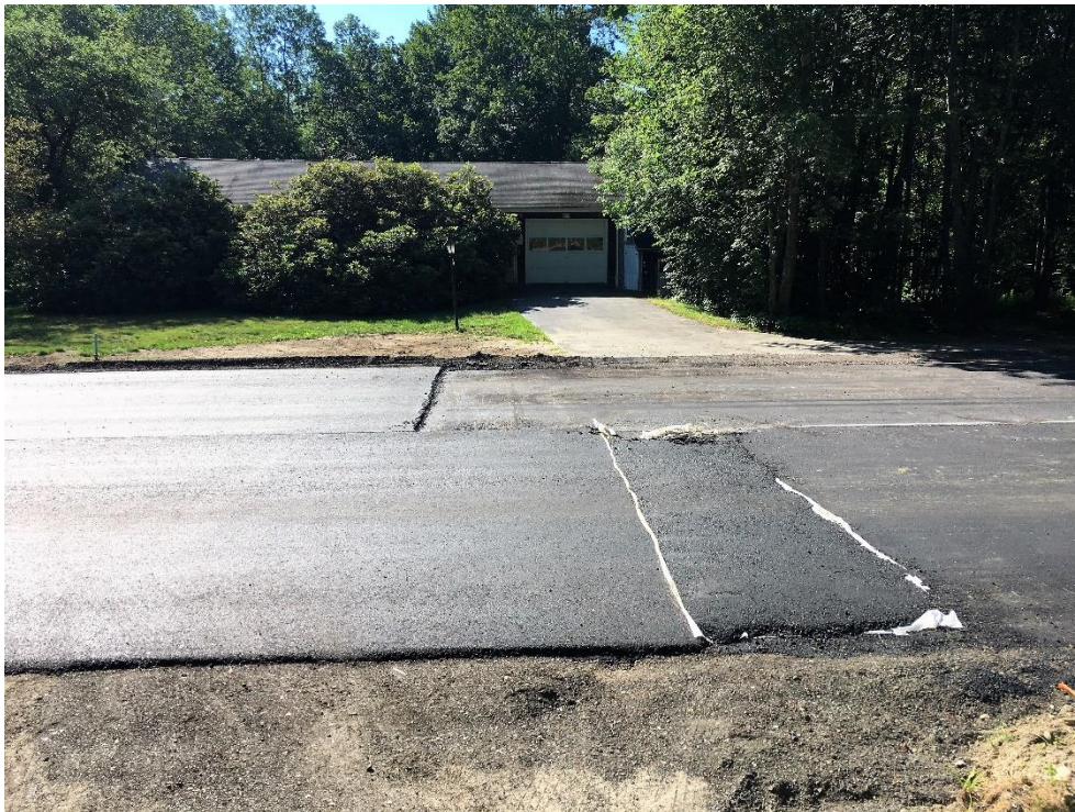
Temporary pavement ramp at STA 79+00 removed in the northbound lane being paved but remaining in the southbound lane until paving switches to southbound lane.
